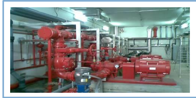
Pump Room Plant
